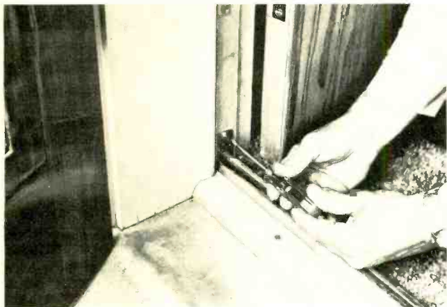
PUSHBUTTON SWITCH INSTALLED inside a door jam will detect anyone opening the door. This switch is part of a Westinghouse system.
