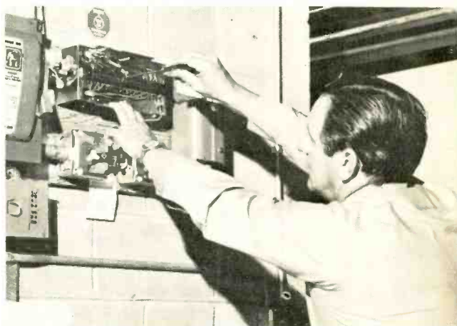
MULTISTATION ALARM INSTALLATION may call for a central control box. A Westinghouse system is being installed here.
